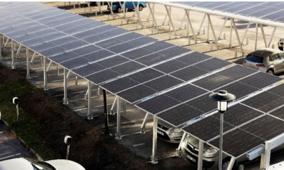
Solar carports at Scandic Luleå
