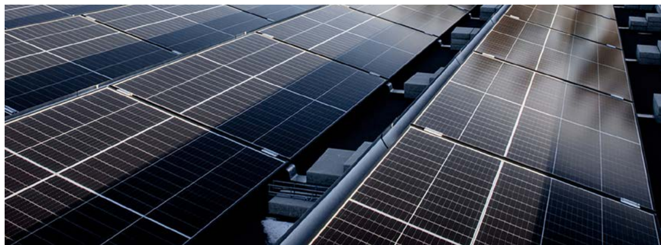
The solar panels at CTT Bribo were commissioned at the end of 2021 and produced around 220,000 kWh in 2022. Above expectations of 200,000 kWh.
