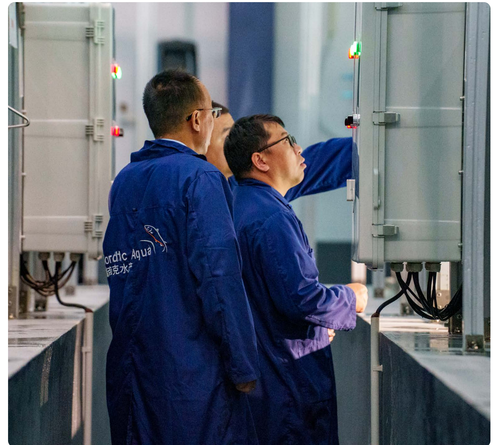
Monitoring and control of energy systems at the Group's Ningbo RAS facility
