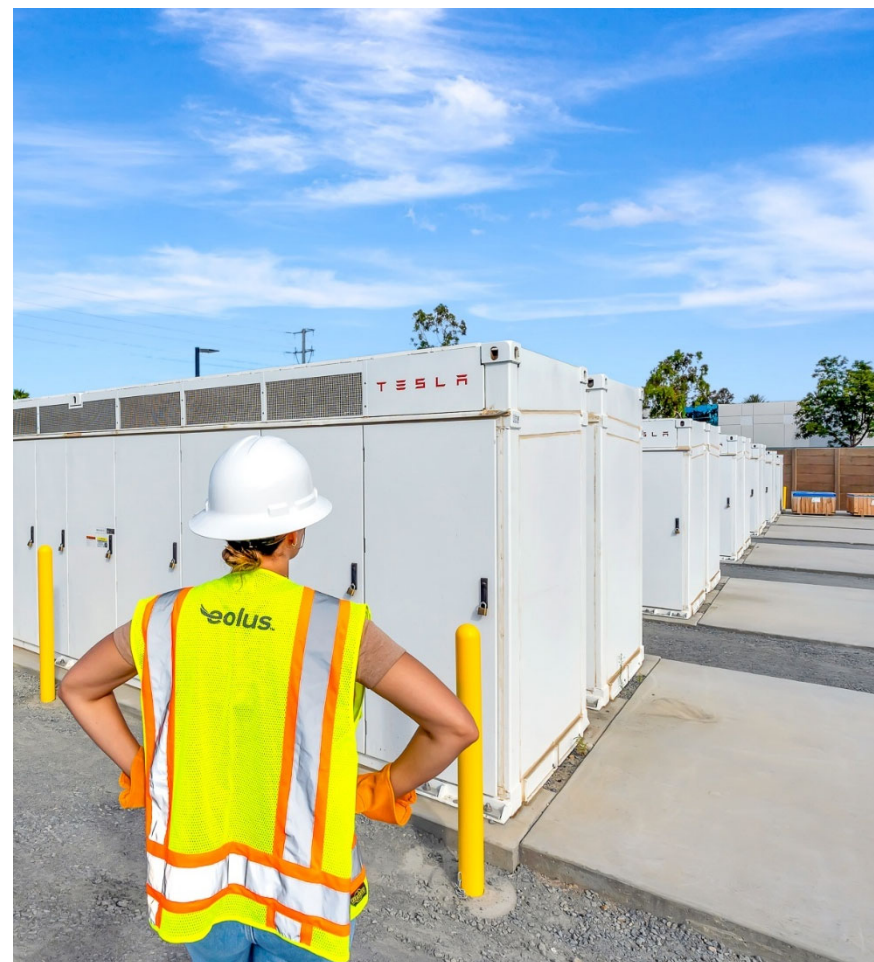
The Pome battery storage project in Poway, California, comprises 100 MW. Eolus sold the project in January 2025 to a leading privately owned US renewable energy producer but continues to lead the construction on behalf of the buyer.
