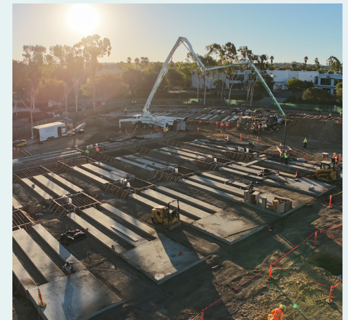
Pome is under construction on a 16 000 square meter plot in the urban San Diego area.
