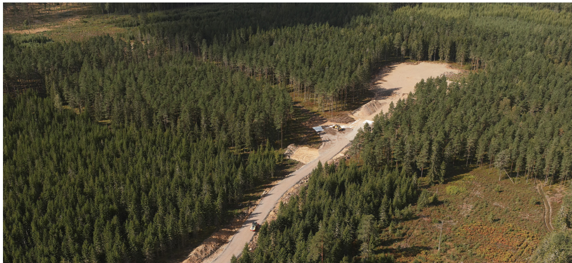
Construction of Fågelås Wind Farm in Hjo. The project comprises seven wind turbines with a total installed capacity of 45 MW.
