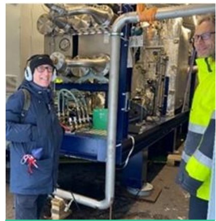
Landmark Power Holdings' CEO, Michael Avison, at a demonstration of HeatPower 300 during a visit at Climeon's test site in Kista.
