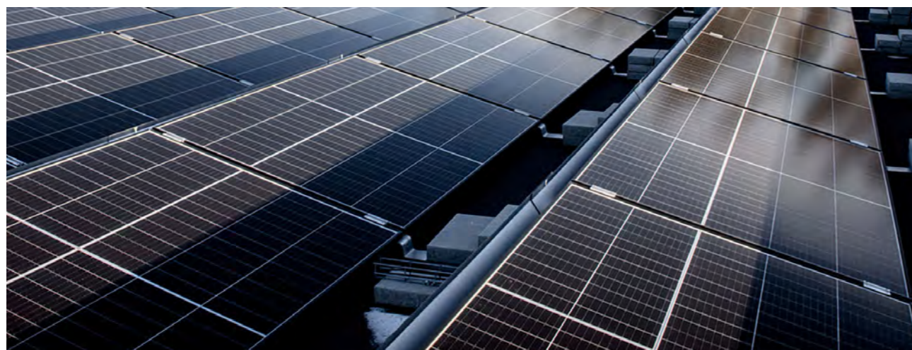
The solar panels at CTT Nybro were commissioned at the end of 2021 and produced around 205,000 kWh in 2023. Above expectations of 200,000 kWh.
