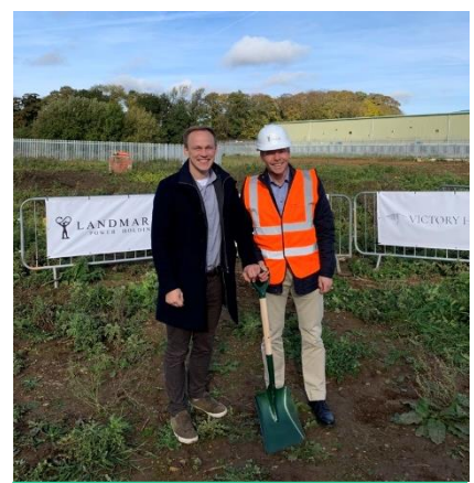
Climeon's team members attended the ground-breaking ceremony for the start of construction on a low-carbon flexible power project in Rhodesia, Worksop, UK.
