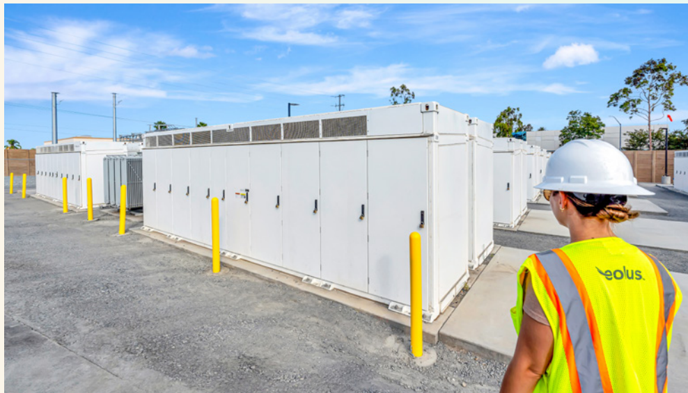
The Pome battery storage project in the San Diego area was completed in 2025. Read more about the project on page 36.
