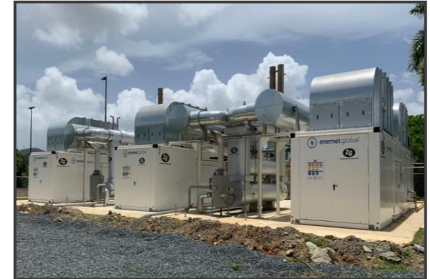
Neol CHP Puerto Rico Overall progress: 100% Final Testing
