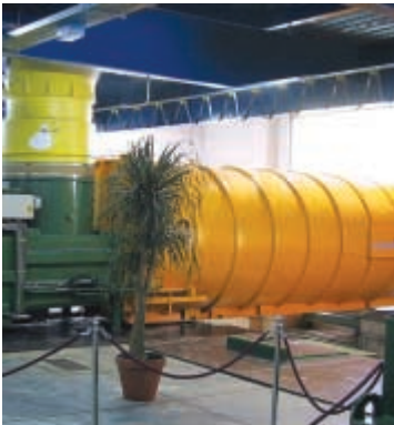
Envac operates within waste management. The picture shows a reception station in Seville, Spain.
