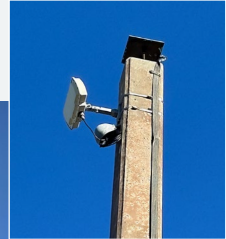
RTMS Echo – radar-based detection technology installed in Tampa, Florida, USA.
