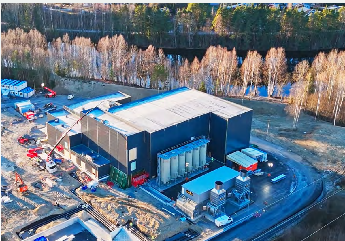
The large-scale Hønefoss project shaping up with buildings and infrastructure largely in place.
