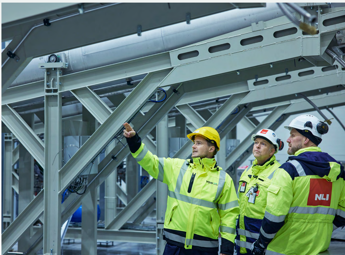
Installation of process equipment at the large-scale Hønefoss facility commenced in October 2024.
