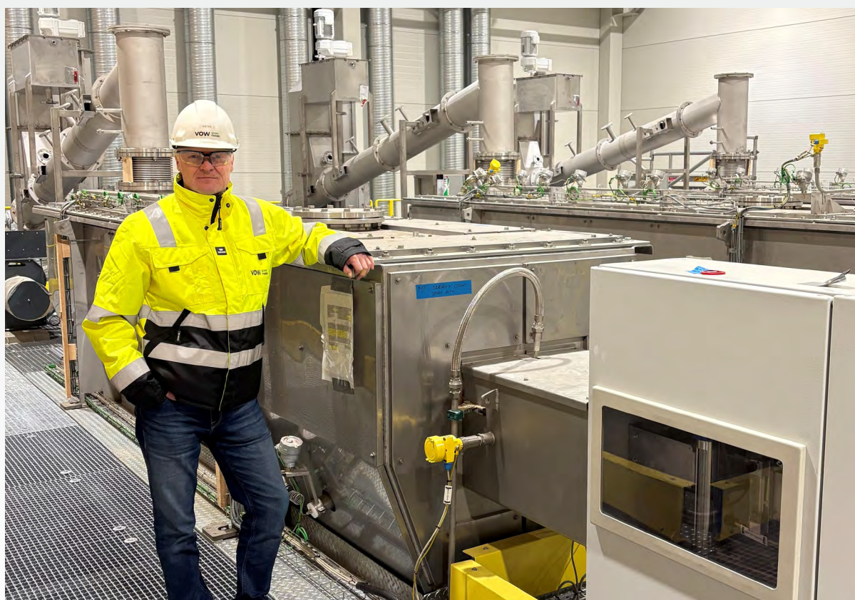
All four pyrolysis reactors successfully installed inside the pyrolysis hall of the large-scale Hønefoss facility.
