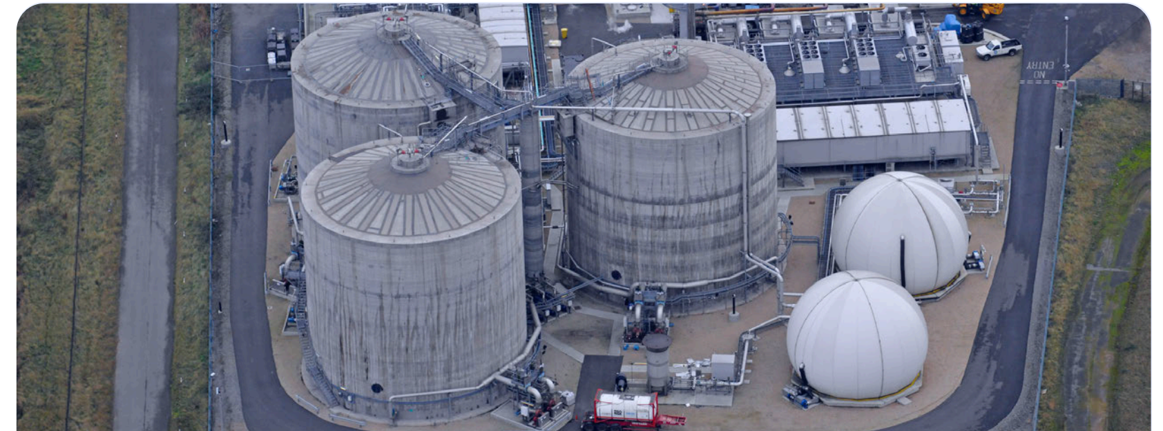
Cambi THP system in operation at modern bioresources hub in the UK
