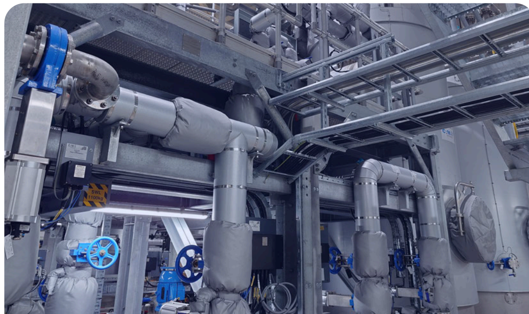
First THP system model E in operation in Lillestrøm, Norway
