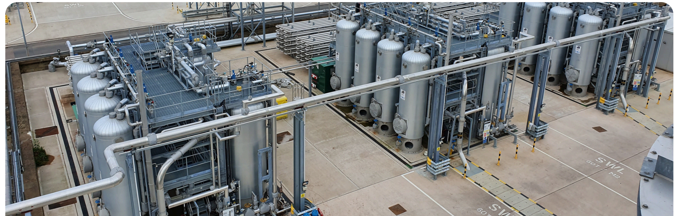
Three Cambi THP systems in operation in Birmingham, UK
