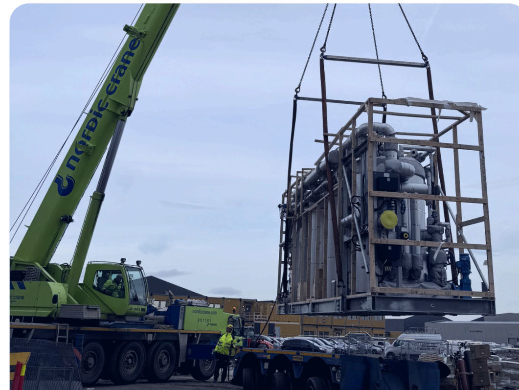
THP system delivery in Fredrikstad, Norway
