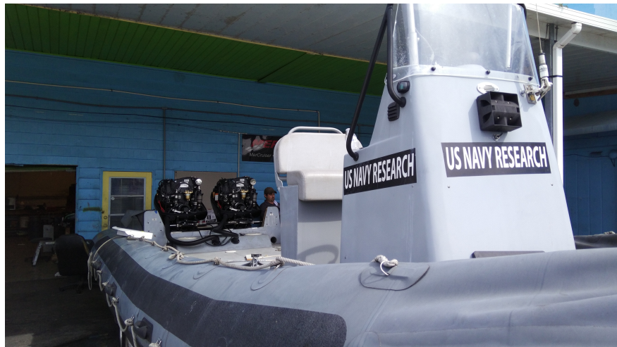
Figure 3 - Installation of the twin OXE 150hp at the US Navy research centre. They were happy with the initial trials and commented that there was little difference in top speed when compared to the 200hp
