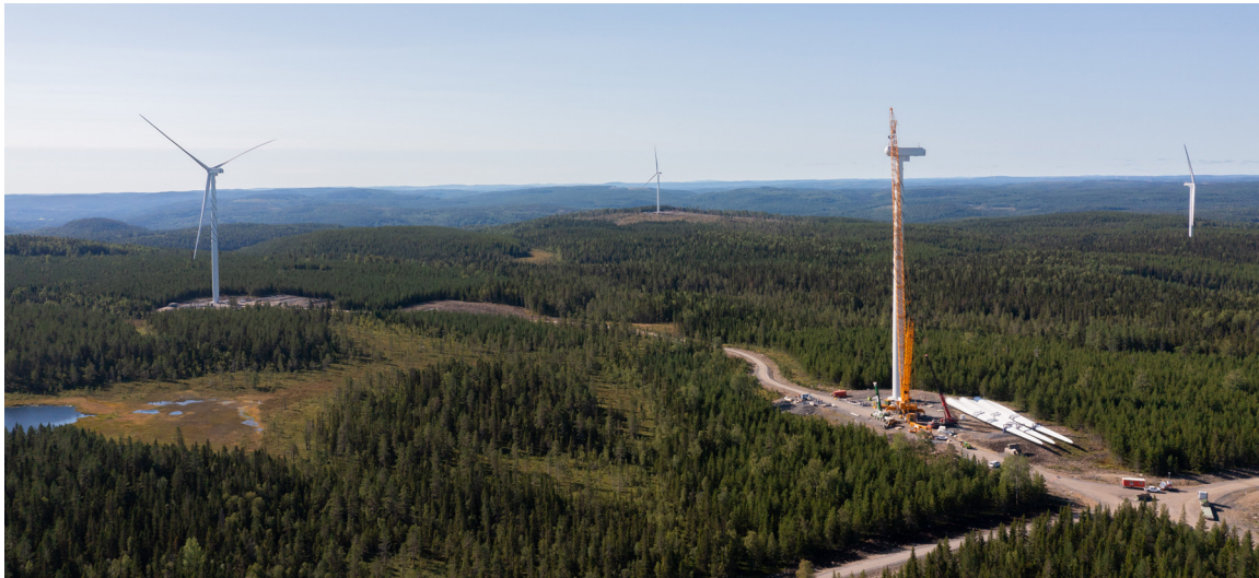
The construction of the Stor-Skälsjön wind farm, with 42 turbines and 260 MW of installed capacity, is in its final stages.
