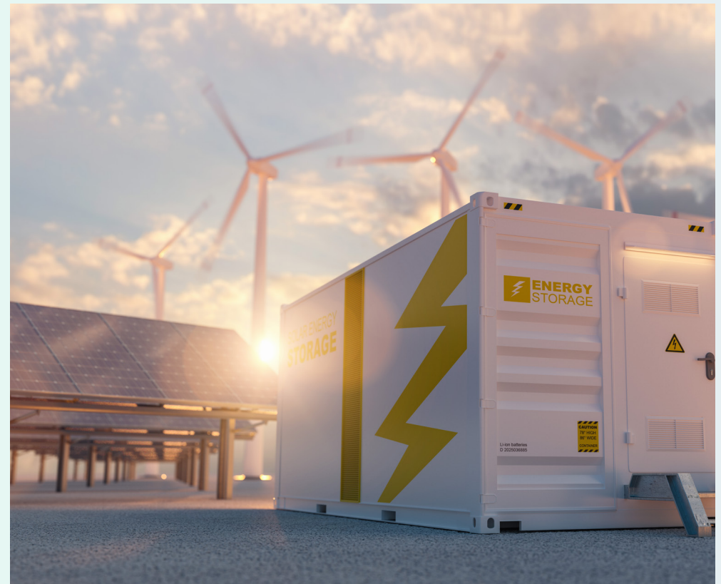
Battery storage can be established either as stand-alone installations or together with wind and/or solar power.
