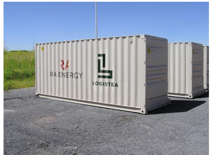
Illustration of the batteries in Vaggeryd Logistikpark.
