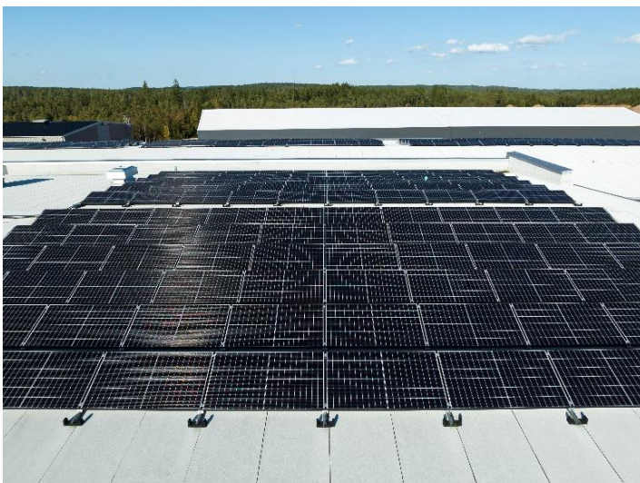
Solar panels on the property Lockryd 2:73 in Svenljunga
