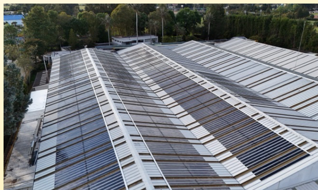
The installation on the roof of Yazaki's facility in Bogotá comprises 872 panels with a total capacity of 144 kWp.
