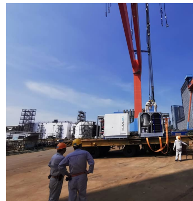
In July, the integration of Heat Power modules onboard Viking Line's new ship, Viking Glory, began.
