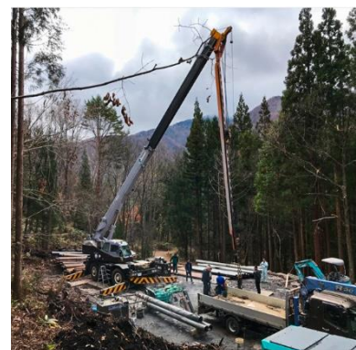
Climeon's customer Baseload Power Japan has started drilling on the first sites.
