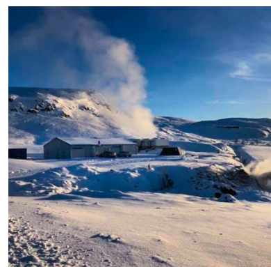
Varmaorka is conducting final tests of their first geothermal heat power plant, including Climeon's Heat Power modules.
