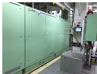
Climeon Heat Power system on board Virgin Voyage's ship.
