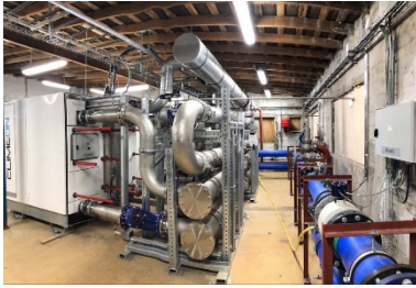
Climeon modules shown at Varmaorka's Reykholt power plant.
