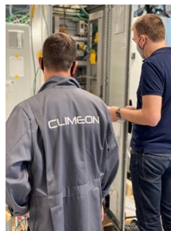
Inspection in the test site. DNV approves the remaining modules for Havila Voyages
