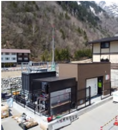
In Japan, installation work is underway at two different power plants, one of which was commissioned at the end of April.
