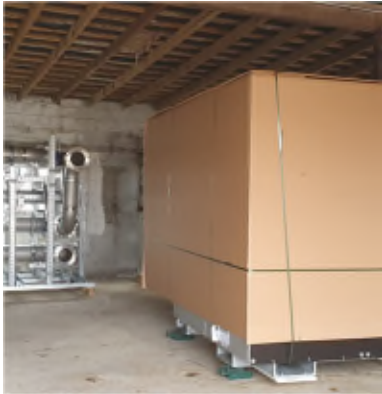
In Reykholt, Iceland, Climeon has started the installation of the Heat Power systems and the company's prototype for standardized pipelines, the Backbone.
