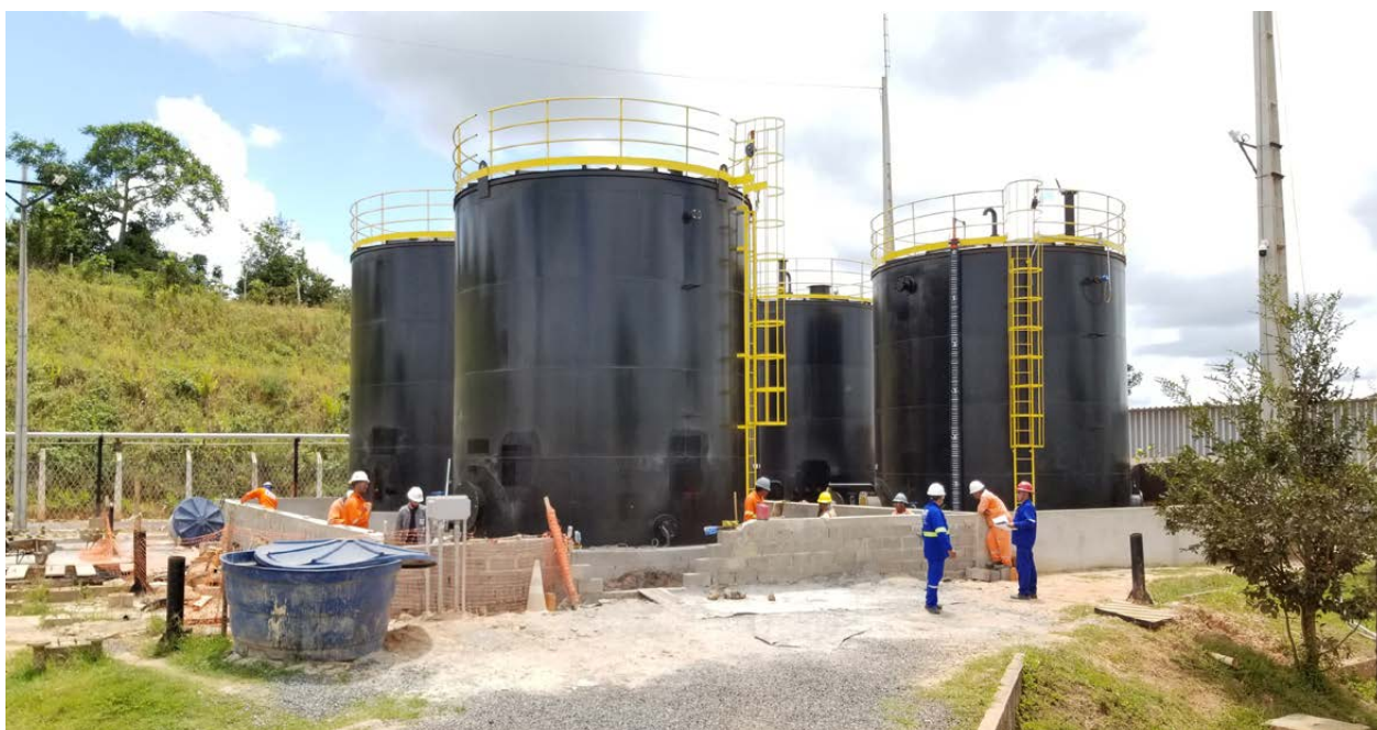
Four new 1,000 bbls oil storage tanks
