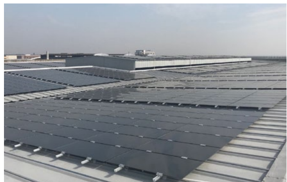
Shaoxing Longze Pipeline Co. 1,43 MW
