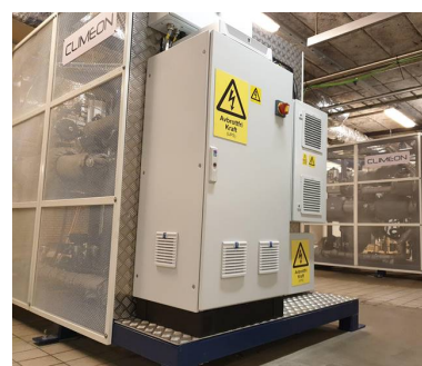
Climeon has developed and delivered two steam turbines to Viking Line's newbuild ship Viking Glory.
